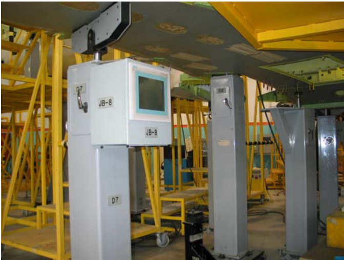
Figure 38. Screen display location in the join cell, looking inboard
